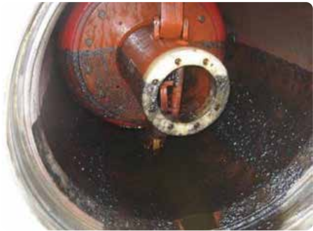
Figure 1. Result of pigging a “dry” network
