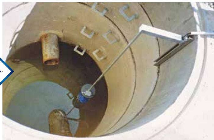
Monitoring in an Unmanned Pumping Station
