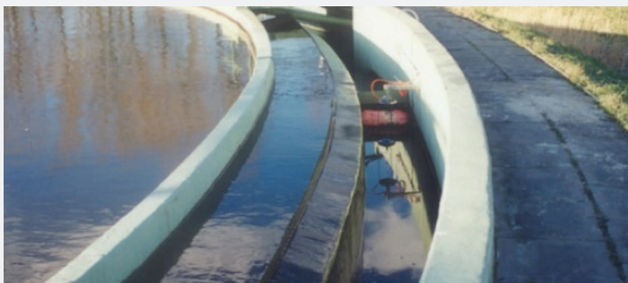
ID-223/500 Monitoring Water Discharge from a Gravity Separator
