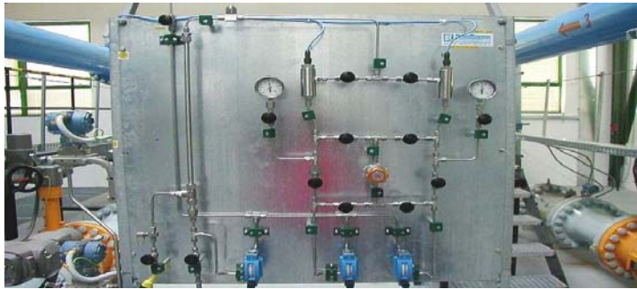
Figure 2. Natural gas compressor dehydration station – (Transport natural gas moisture analysis)
